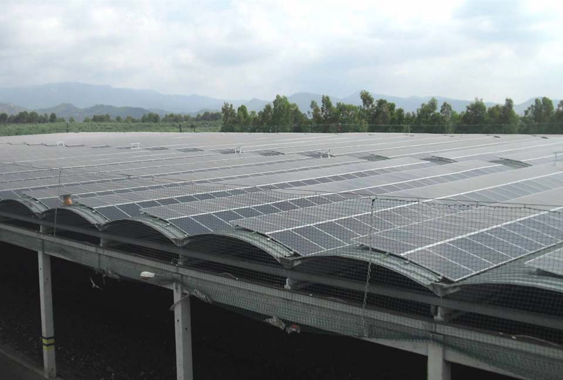
Centre Residus de Botarell, Reus – 2.376 kWp
